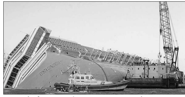
A sea platform carrying a crane approaches Costa Concordia off the Tuscan island of Giglio, Italy.
